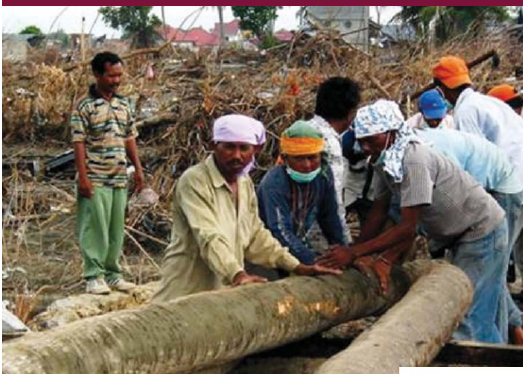
This Mercy Corps project built a temporary bridge to replace infrastructure destroyed by the tsunami.
