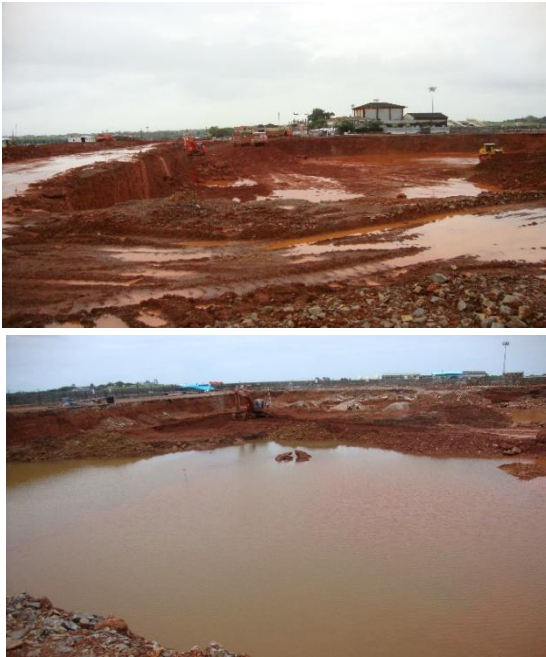
Project site picture demonstrating excessive water-logging on site due to heavy unseasonal rainfall
